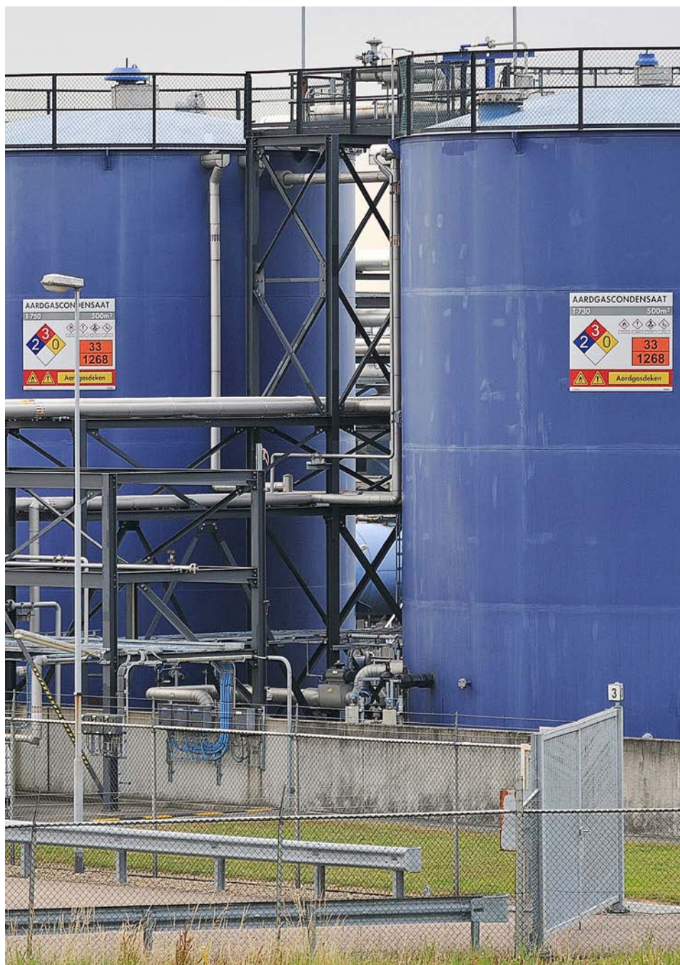
PGS 29 tanks in Gaag (foto SodM)
